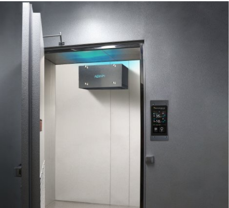
Upper-air UV-C disinfection fixture and environmental control monitor installed in a walk-in cooler environment used in third-party microbial testing. Photo courtesy of Everidge.
