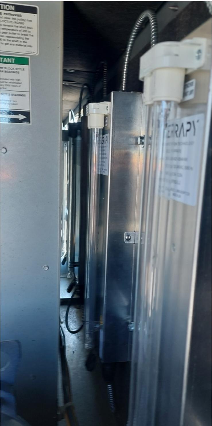
UV-C lamps in continuous operation at the cooling coil of an air-handling unit in a meat-processing facility. Properly engineered HVAC UVGI systems can support both airborne microbial reduction through repeated air treatment and coil-surface hygiene that helps preserve heat-transfer efficiency, reduce pressure drop, and lower HVAC energy demand over time. Photo courtesy of Aerapy.
